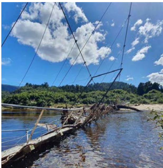
Damage to the Heaphy Bridge. Photo: DOC
